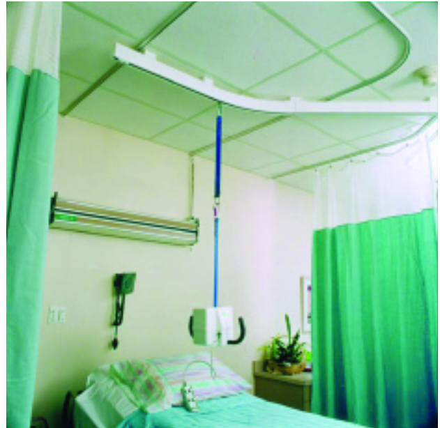
Waverly Glen Hospital Ceiling Lift
